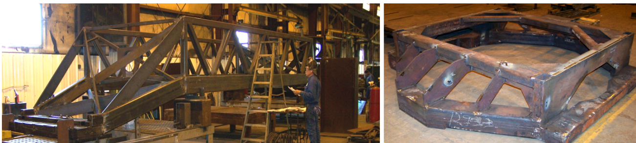
Figure 4. Photographs of the tracker bridge (left) and carriage (right) weldments during fabrication.
