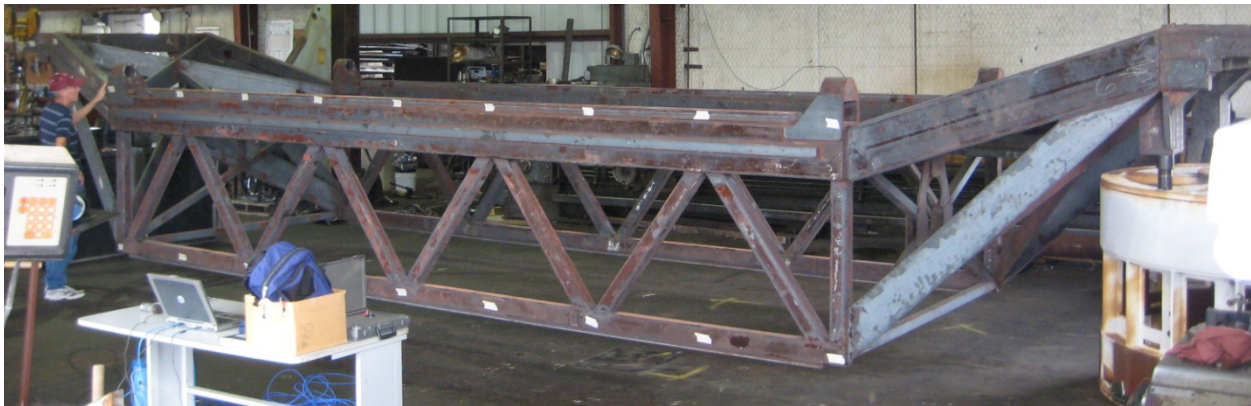
Figure 11: Photograph of the bridge after completion of fabrication and stress relieving, prior to machining
